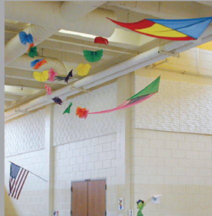
Elementary school's multipurpose room has SONEX® One Panels installed to improve learning environment
