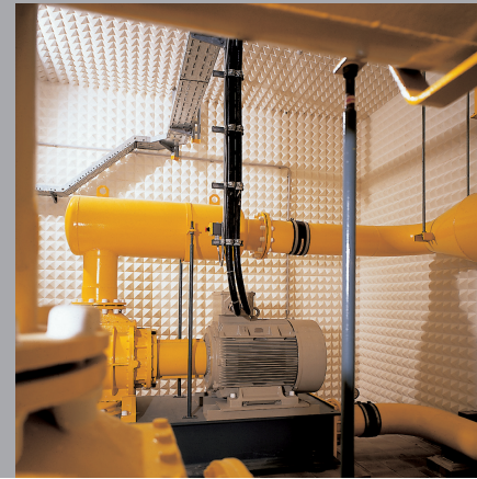
SONEX Pyramid panels used in a manufacturing facility
